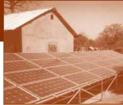
Autonoom PV-systeem in Gambia (Solar Technics)
